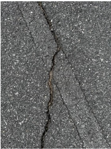
Stripe vs. Asphalt Crack
